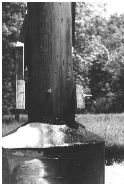
Photo 33. Tower pole and concrete collar connection. Note taper of concrete. Photo courtesy of Mr. Tibor Latincsics.
