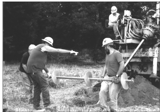
Photo 36. Pete Morrissey directing the helical anchor installation by Trail Conference and GPU Energy volunteers. Photo courtesy of Mr. Tibor Latincics.
