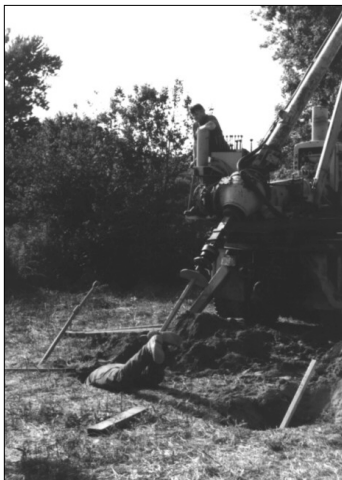
Photo 39. Pete Morrissey bolting the coupling between the two halves of the six helix anchor. Photo courtesy of Mr. Tibor Latincsecs.
