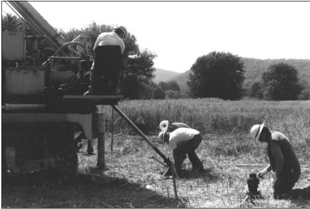
Photo 35. Start of the helical anchor installation. Photo courtesy of Mr. Stephen Klein, Jr.
