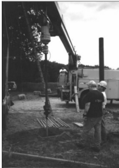
Photo 40. Installation of the Chance® Helical Pier at each corner of the snowshoe foundation. Photo courtesy of Mr. Tibor Latincsecs.
