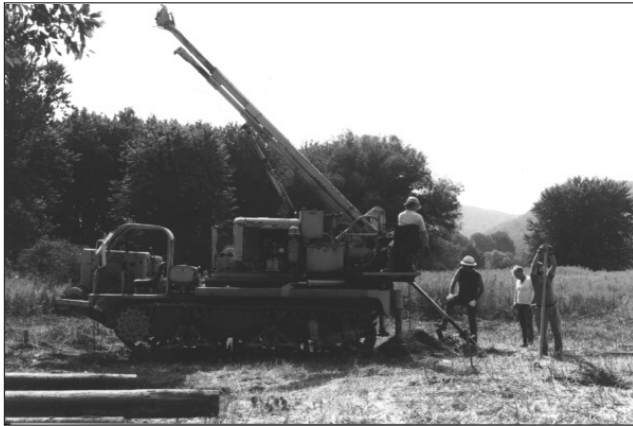
Photo 38. Helical anchors for the backstay anchorage were installed at 46 degrees. Photo courtesy of Mr. Stephen Klein, Jr.
