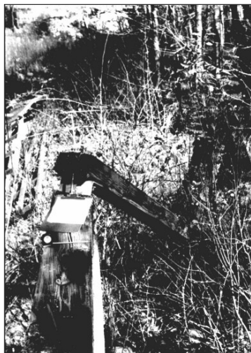
Photo 53. The timber towers were sheared at the base by floodwater driven debris. Photo courtesy of Mr. Tibor Latincics.
