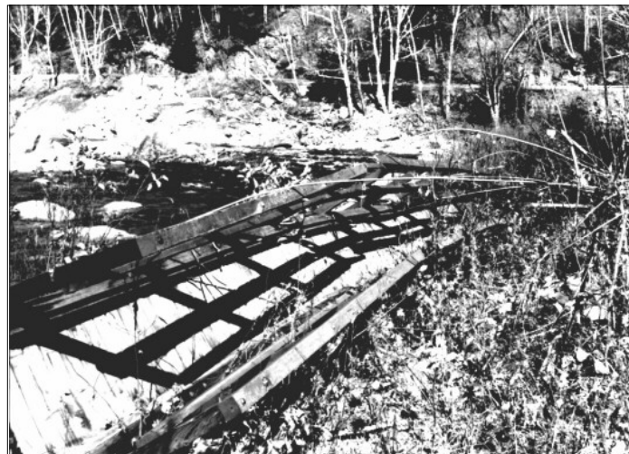
Photo 54. Hastings Bridge walkway remains flung downstream. Photo courtesy of Mr. Tibor Latincics.
